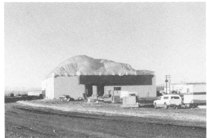
Photo 2 Warm air supported polyethylene tent over the entire roof of a new building being constructed in the winter.
