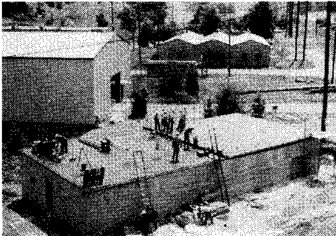
Photo 1 View of RMPRA (looking south). BUR section is on the left. Fully adhered EPDM section is on the upper right. Mechanically attached EPDM is on the lower right. Small, low building is the RTRA.
