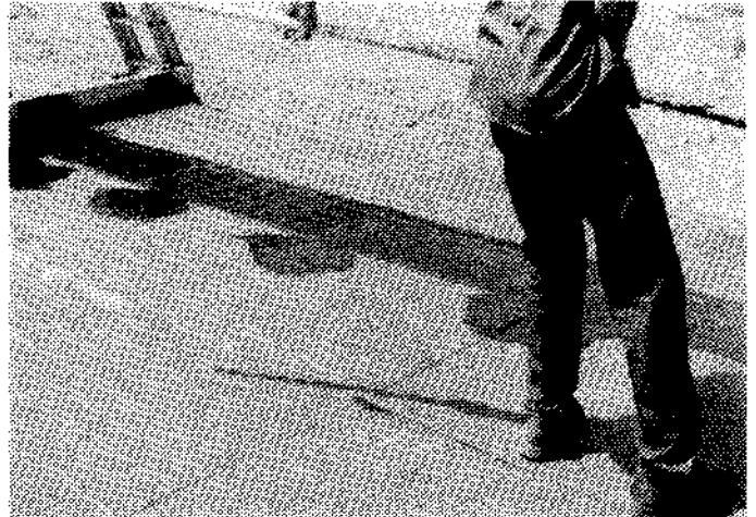
Photo 3 The base sheet was attached with spot mopping of asphalt in the field of the sheet. At the laps, the mopping was continuous as shown.
