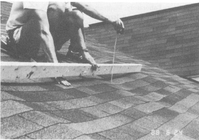
Figure 2 Excessive deflection of FRT plywood decking.
