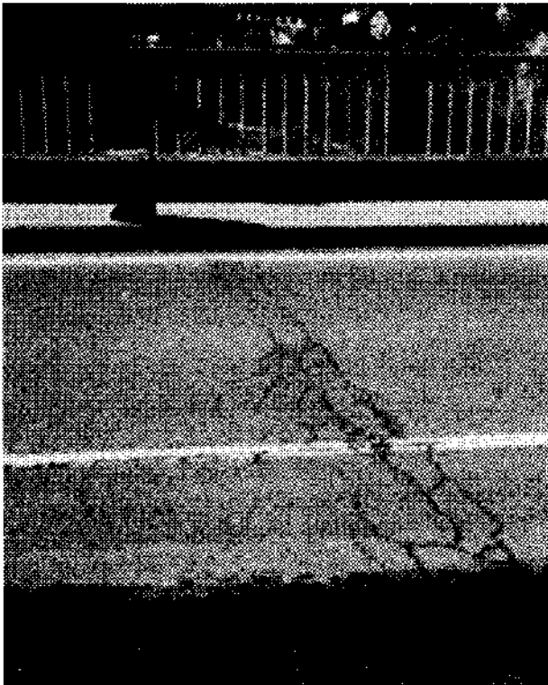
Figure 20: Cracking in asphalt layers at subsurface joint area
