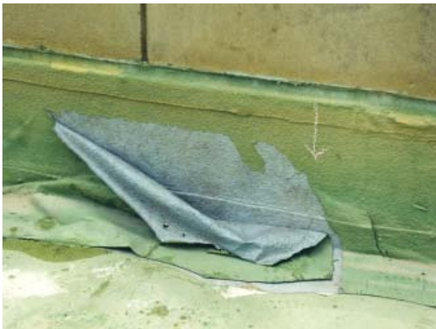
Figure 6 – Large interlayer delaminations of the membrane.
