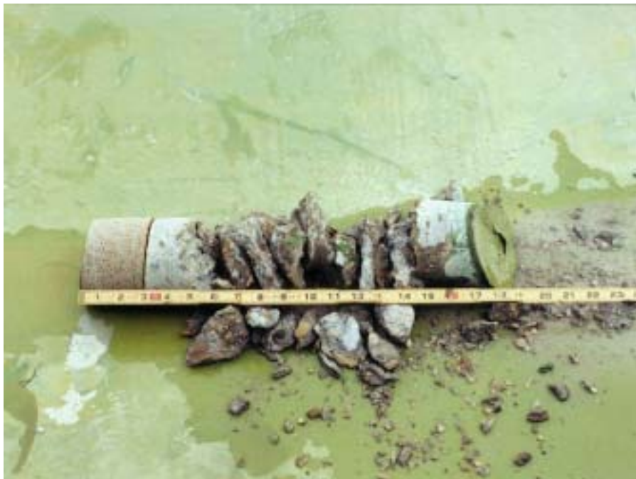
Figure 10 – Core retrieved from a wall section revealed extensive delaminations in the center portion of the wall. The outer layers do not exhibit delamination.
