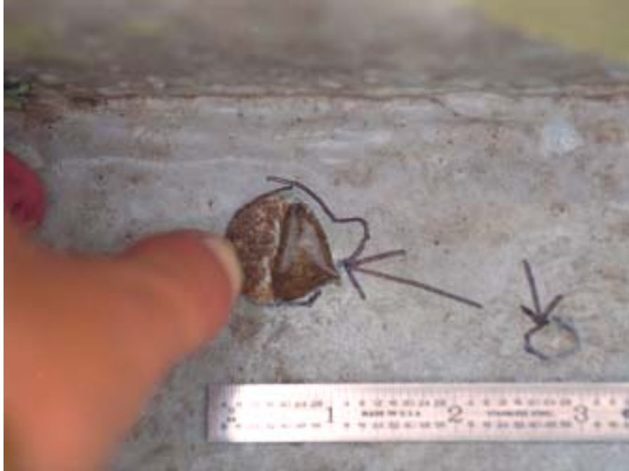
Figure 3 – Water entrapped in the blister shown in Figure 2.
