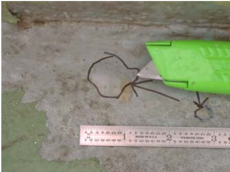
Figure 2 – Water-filled blister in a liquid-applied membrane.
