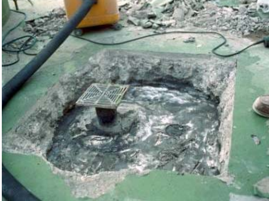
Figure 11 – Overall view of Opening 1 showing the original lead pan and a retrofit drain.
