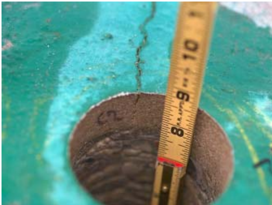
Figure 8 – Substrate crack reflecting through the membrane.
